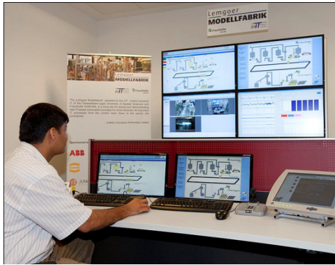
Figure 5: Example of a Control Room (by RobertRED, http://de.wikipedia.org/wiki/Leitstand retrieved February 9, 2011)
